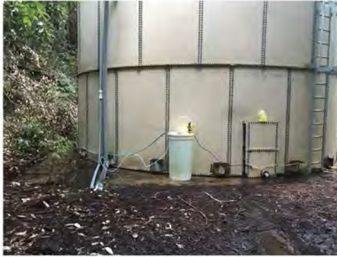
Figure 1. Temporary Disinfectant Injection Configuration at Well # 4
