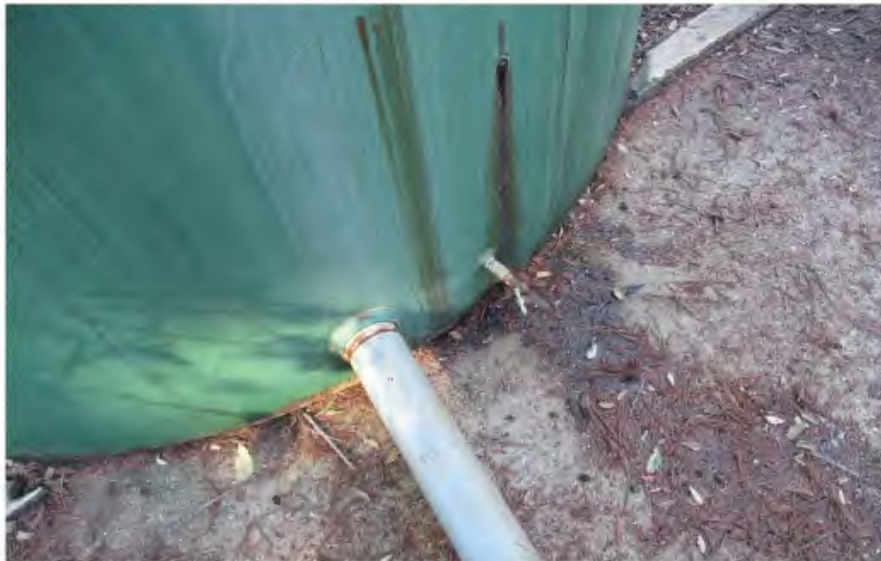
Corrosion and Leaks in the Tank Sidewall
