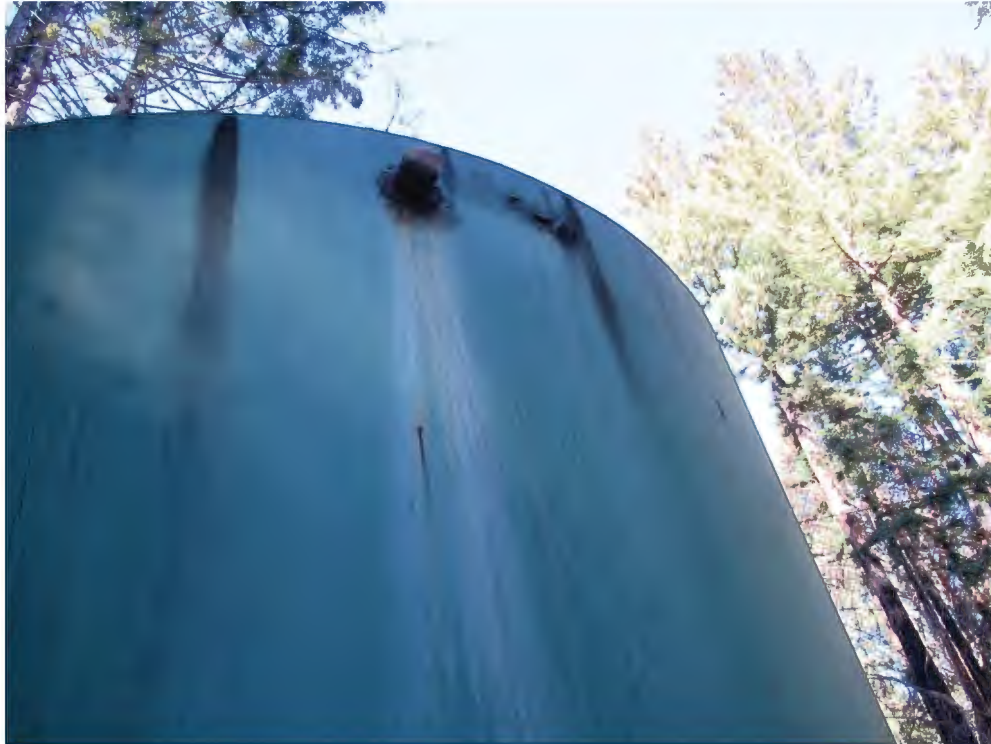
Holes in the Tank Sidewall
